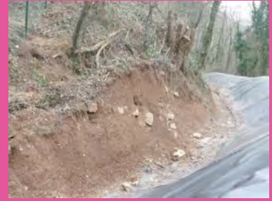
Picture 1-2-3 : Slopes and embankments prone to erosion
